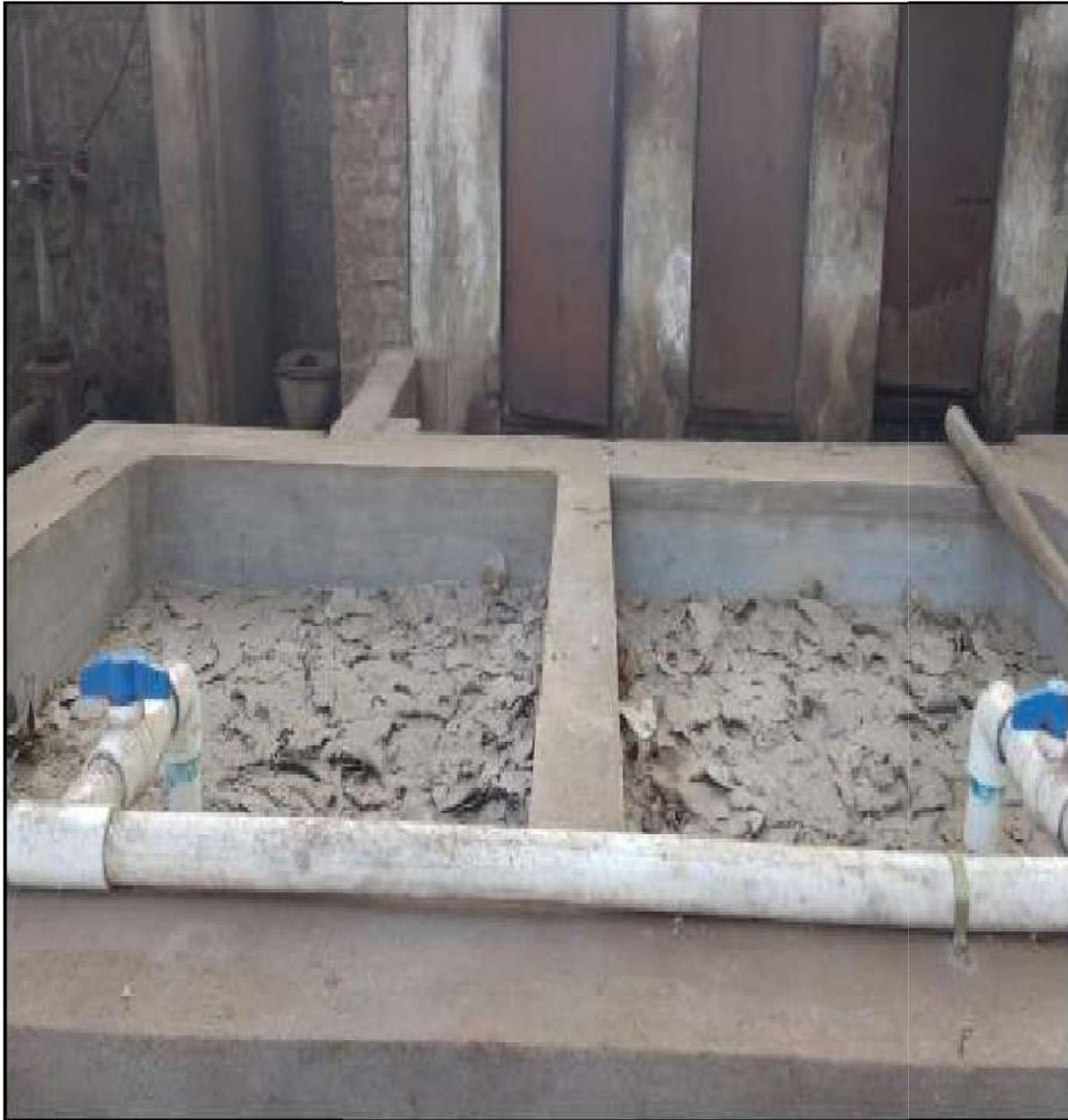
SLUDGE DRYING BED
